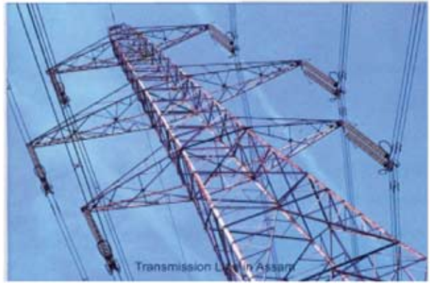
Transmission Line, Assam
